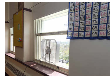
Window fans for ventilation
